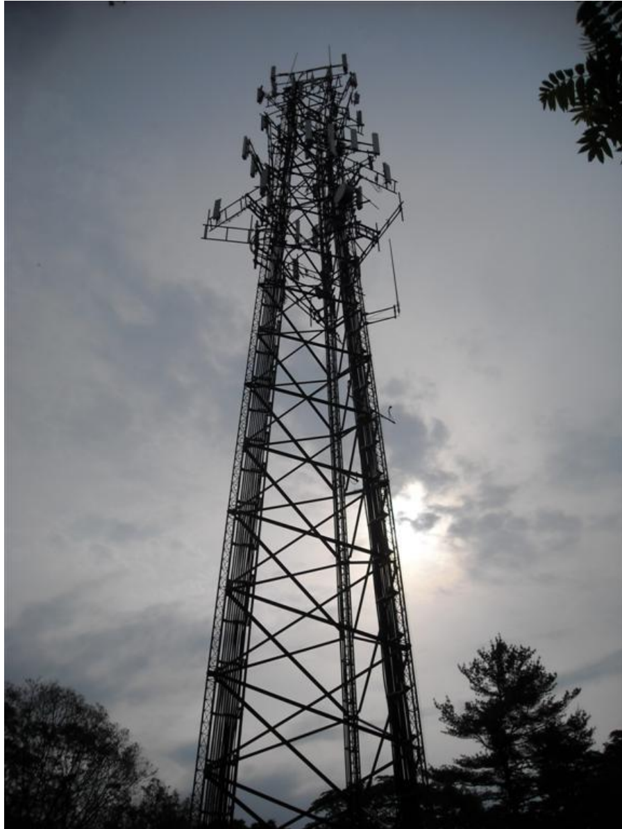
Overview of 160' self-supporting tower.
