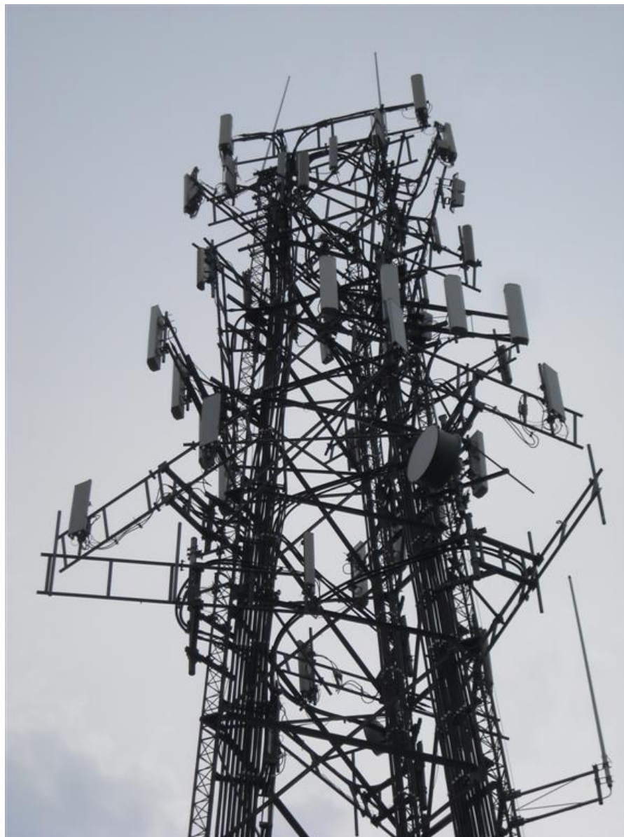
Photo showing existing antennas.
